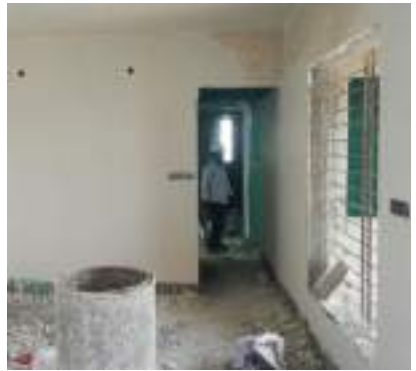
YASHWIN ENCORE - 'B1B2' WALL GYPSUM WORK IS IN PROGRESS ON 18 TH FLOOR.
