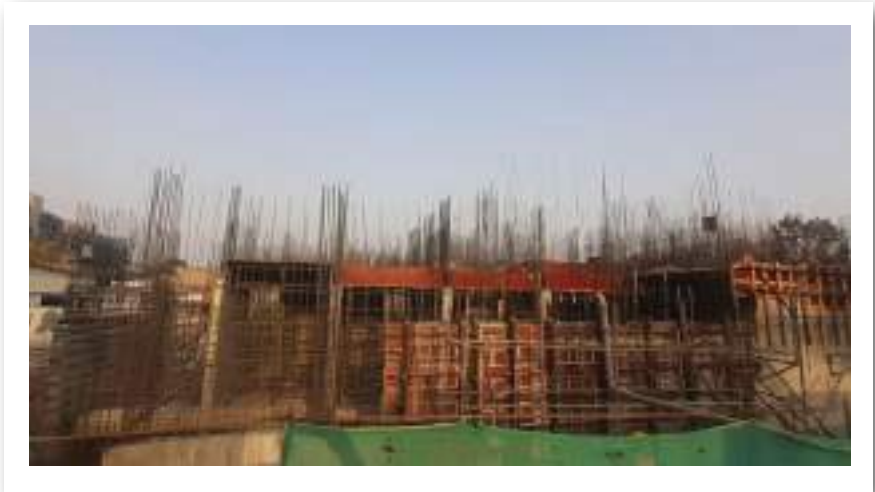
YASHWIN ORIZZONTE - 'B' NORTH SIDE SHUTTERING WORK IS IN PROGRESS FOR 1 ST SLAB.
